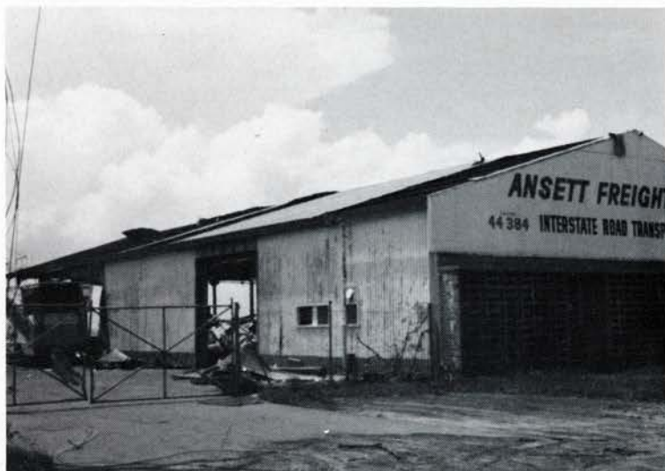
Angled shot of old AFE depot now being used for Wridgway storage. Most of the front and southern wall were left intact but most of the roof, western and northern walls were missing.
