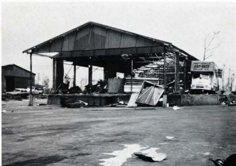
Close up of damage to the rear of the Wridgways building.
